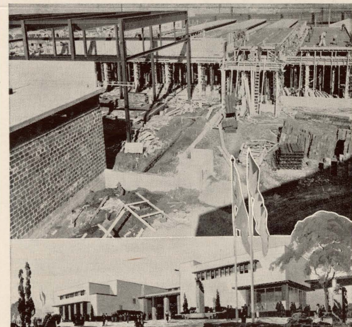
Four processes of building—pouring forms, erecting steel, erecting walls and stuccoing—is under way on Hall of Livestock No. 2. Sketch shows how it will look completed.
